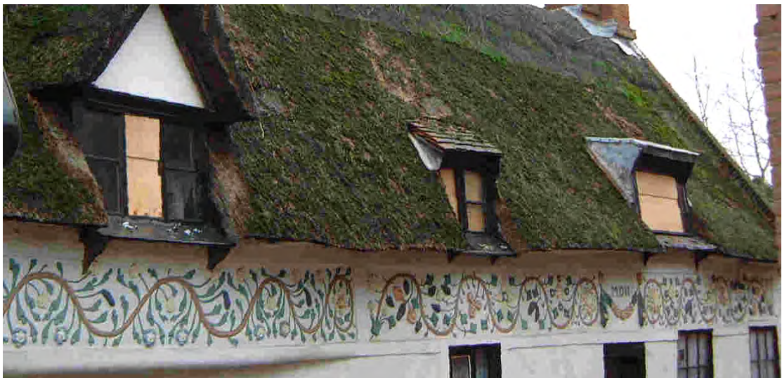
Fig 20. Photograph taken during the repairs to the cottages in 1993-4, the Tudor roses (left side panel at the bottom) are now painted blue and white.
