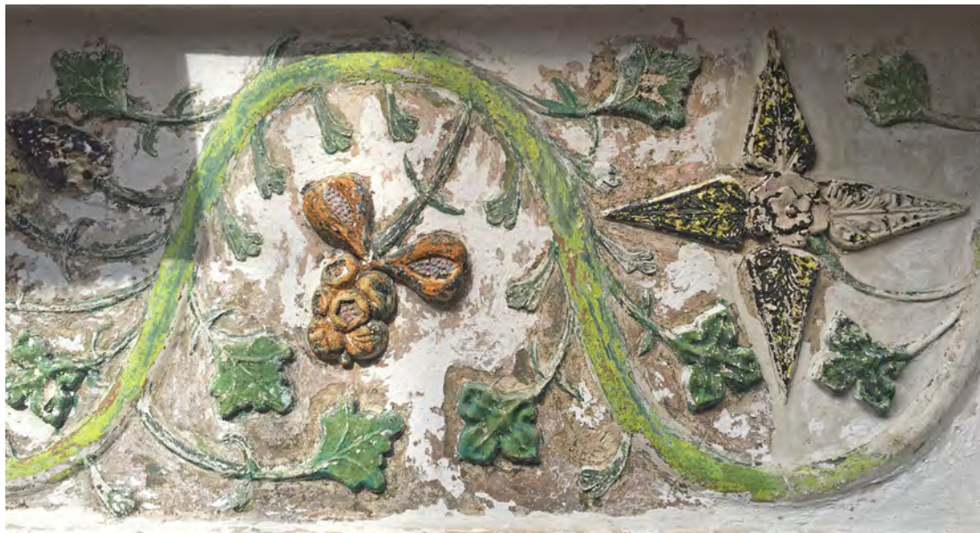
Fig 25. August 2020 The paint stripping revealed the yellow green stem from the 1963 – 1978 colour scheme and the black paint described in 1949.
